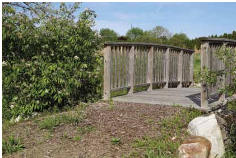
A bridge over an ephemeral stream, created when natural springs were revealed on the site and designed as a central feature of The Preserve.
